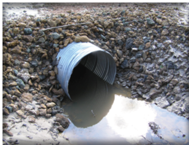
Culvert crossings should be properly sized and armored to prevent them from washing out.
